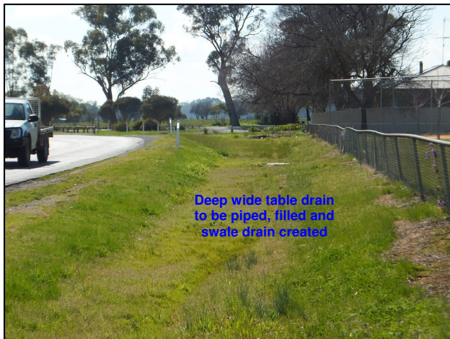
Photo 6 shows existing section of Lookout Rd with deep wide table drain to be filled, piped and swale drain created as part of Option 1 WSP as described in Section 3.1
