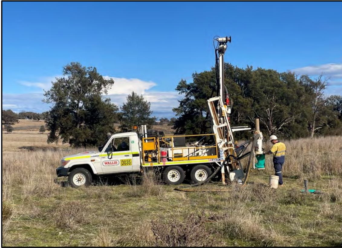
Figure 4: A Wallis Drilling Toyota Landcruiser-mounted Mantis drill rig working for KTA in June 2021.
