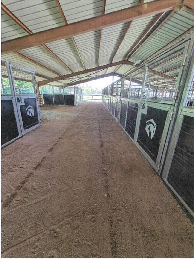
Internal stable alleyways & ventilation
